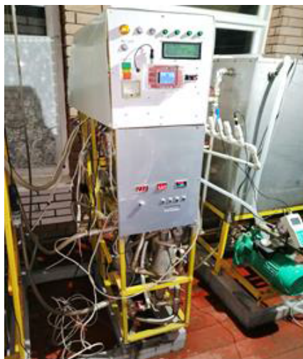
Fig. 1. General view of AWPS
