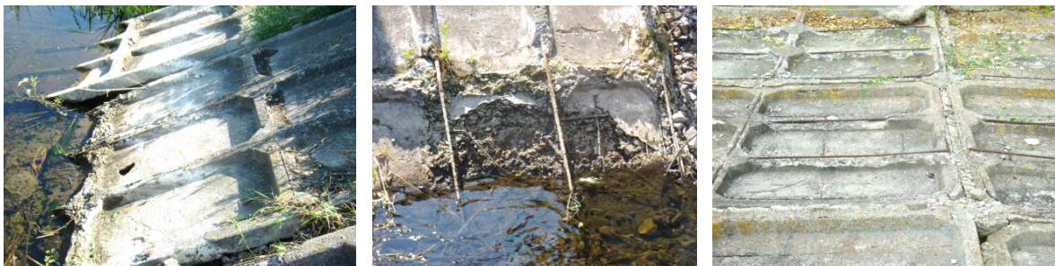
Fig. 2. Technical condition of the pre-chamber panels of the Kochurska pumping station of the Irpin IWMD
