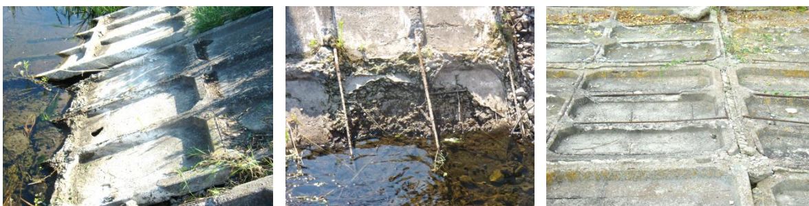
Fig. 2. Technical condition of the pre-chamber panels of the Kochurska pumping station of the Irpin IWMD
